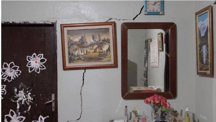
A cracked wall inside the house of former teacher Hilda Ravallito, age 67. These neighborhoods were built by oil companies for their workers. They had their own schools, hospitals and clubs. This site is still legally owned by the state. The houses are falling apart because the ground is sinking, due to its proximity to Lake Maracaibo. © Fabiola Ferrero
