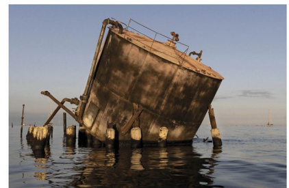
Lake Maracaibo, Zulia, 14th February 2022. An oil tank in Lake Maracaibo. Due to a lack of investment and maintenance over many years, Venezuela's oil production recently hit a historical low, deepening the crisis of a country whose economy depends almost fully on income from oil - Fabiola Ferrero for Fondation Carmignac
